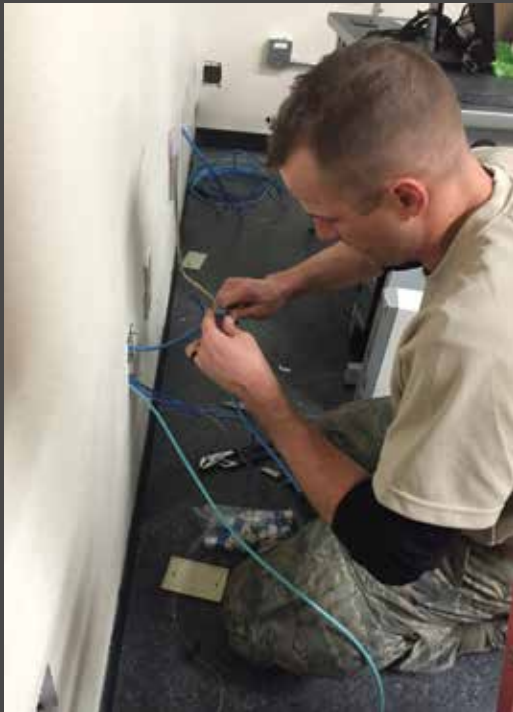
Tech. Sgt. Austin Walje terminating CAT6 wire at Boise Idaho Air National Guard Base.
