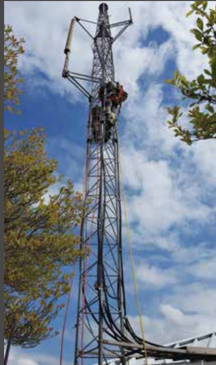
Staff Sgt. Charles Treutlein and Senior Master Sgt. Michael Perez certify on tower climbing during a preventative-maintenance inspection at Portland Air National Guard Base.
