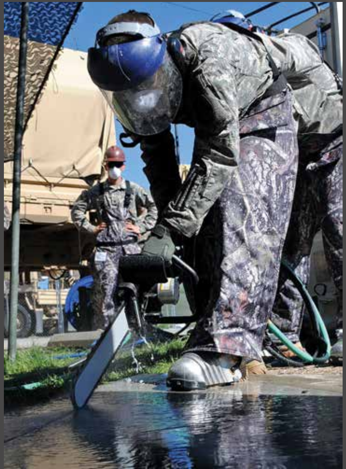
Spc. Kevin Gwilliam from the 624th Engineer Company, 1457th Engineer Battalion, uses a wet saw to cut a section of concrete as part of a renovation project on a restroom facility at the Renegade Point Marina, Strawberry Reservoir, June 8.
